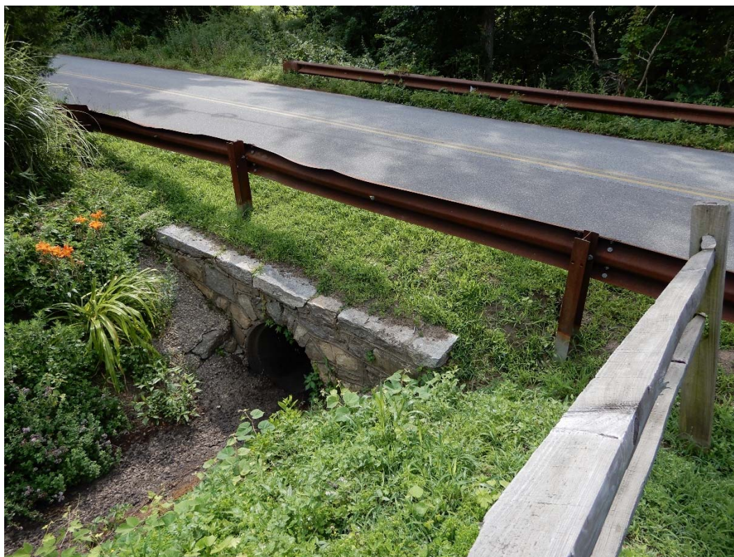
Photo 19b – The upstream end of the left side outlet pipe and headwall.
