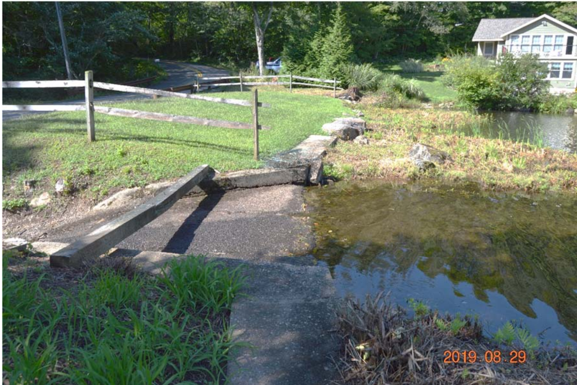
Photo 1a – An overview of Lake Hayward Dam from the left upstream side, with the left side spillway in the foreground.
