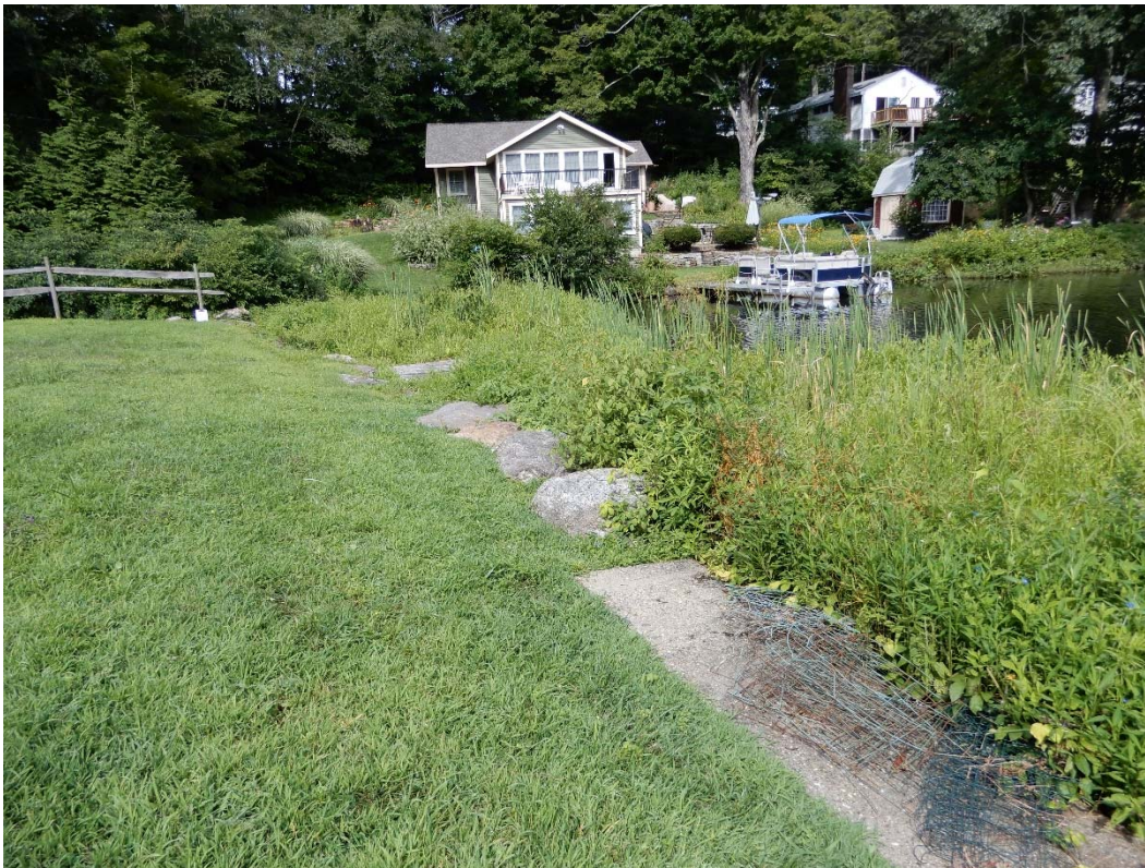
Photo 4a – The upstream embankment as seen from the left side, prior to clearing of vegetation.
