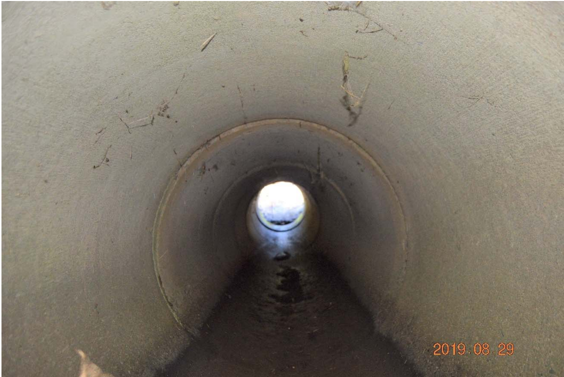
Photo 19g – The interior of the left side outlet pipe, in similarly good condition to the two right side pipes.
