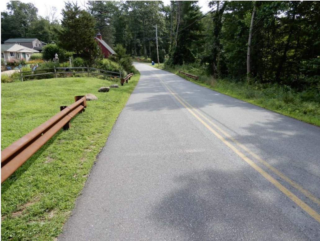
Photo 7b – Another view of the downstream side of the embankment, showing the transition to the adjacent road.
