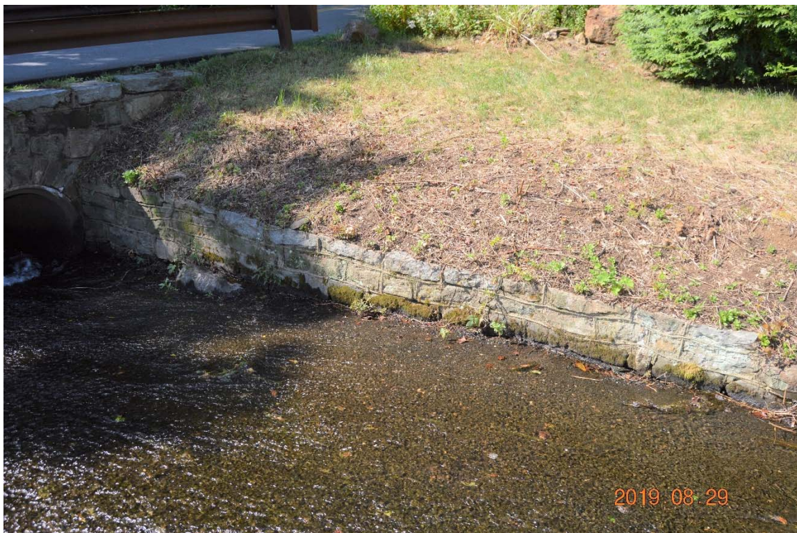
Photo 11a – The right side channel training wall along the discharge channel emanating from the right side spillway.
