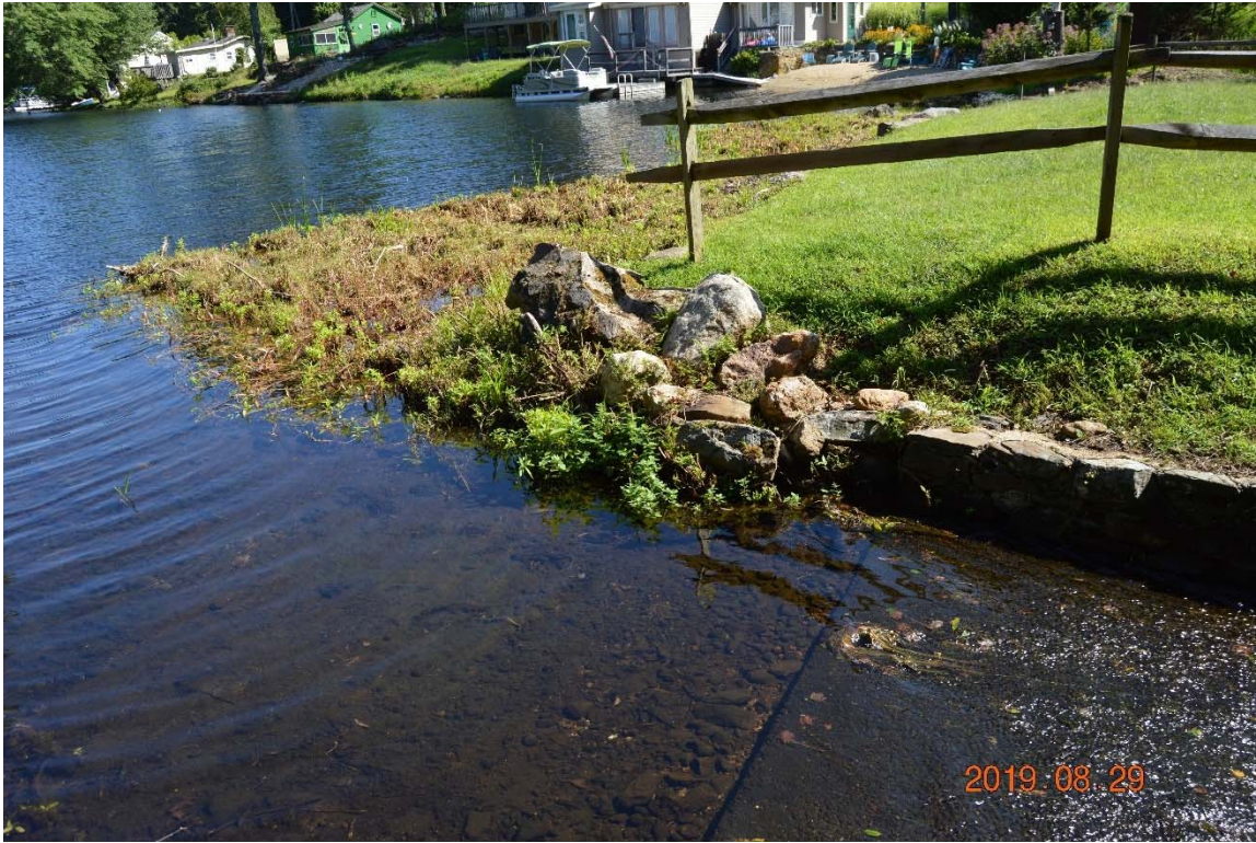
Photo 3d – The junction of the upstream embankment with the right side spillway.
