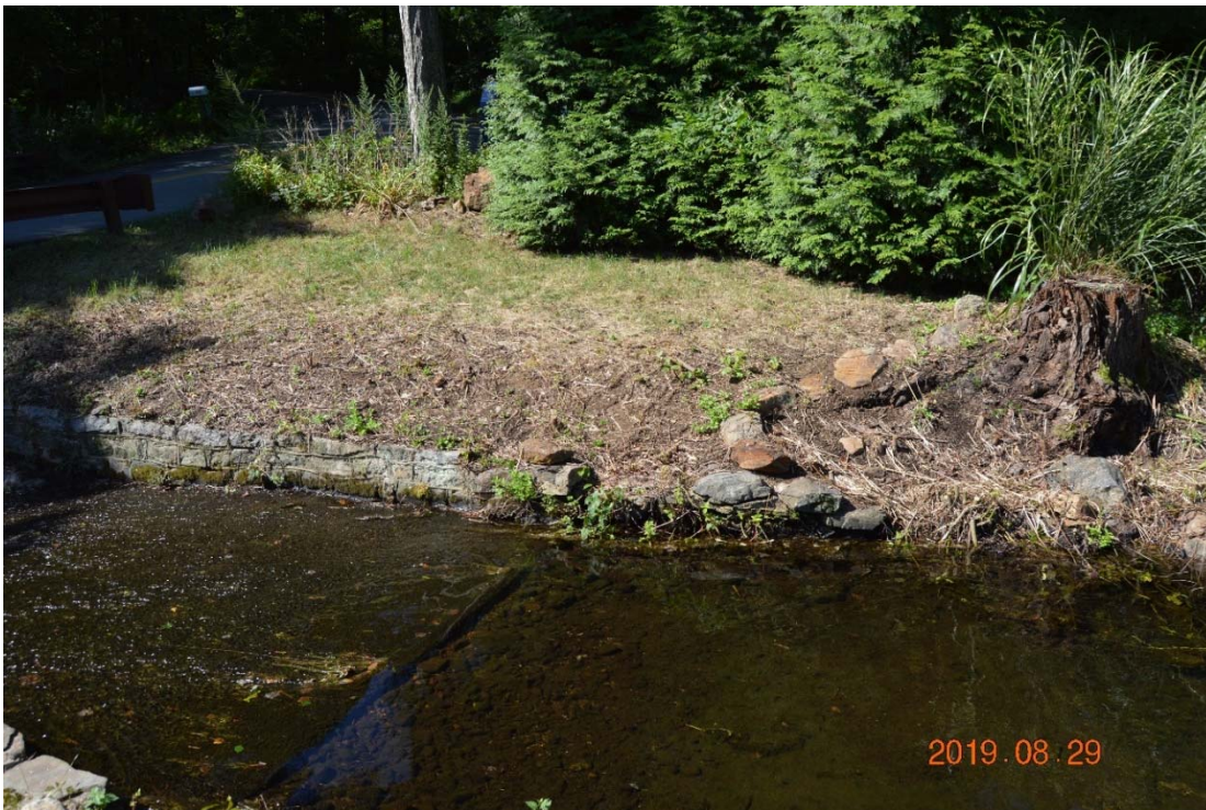
Photo 21b – The embankment along the right side of the right discharge channel. This area was recently cleared of brush and vegetative growth, and should have a grass cover established and maintained. The tree stump (from previous clearing) must be monitored and any depression resulting therefrom filled in as required if subsidence should occur. In the event of reconstruction of the training wall area, the stump and roots should be removed at the same time. The training walls in this area have deficiencies that require improvements and repairs.
