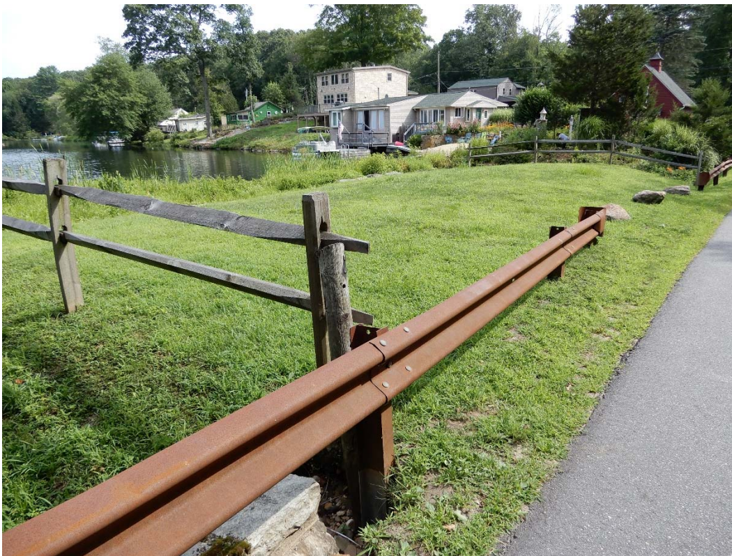
Photo 7a – The downstream embankment face, as seen from the right side discharge culvert.
