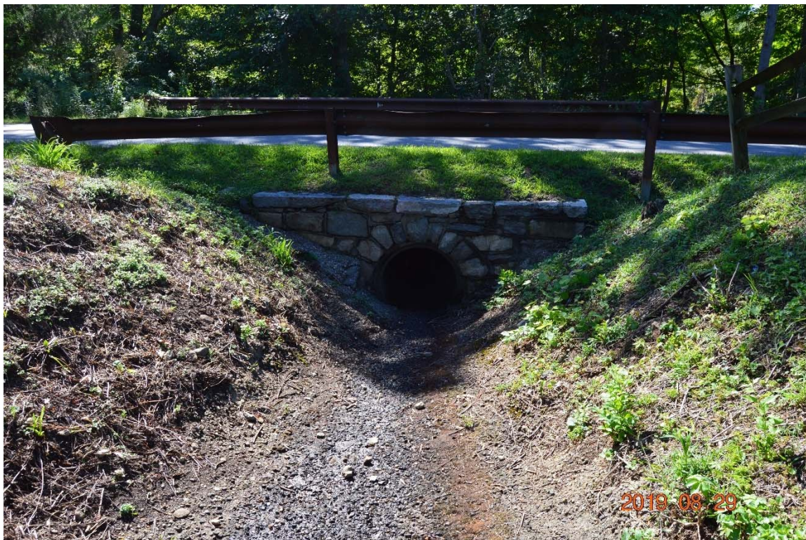
Photo 21f – The lower portion of the left discharge channel. Side slope areas where brush growth was recently cut must be kept cleared with the reestablishment of a grass cover to prevent erosion during high flow situations. (See Section XII for additional long term recommendations.)
