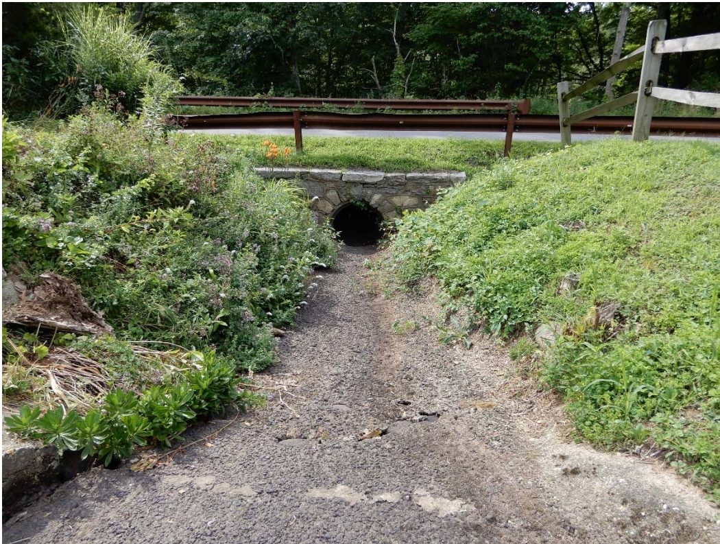
Photo 15a – An overview of the left side discharge channel as seen from the upstream side.
