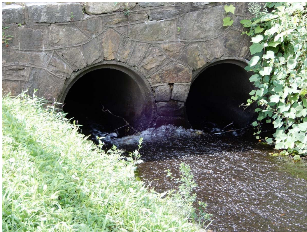
Photo 19a – The upstream end of the right side outlet pipes and headwall.
