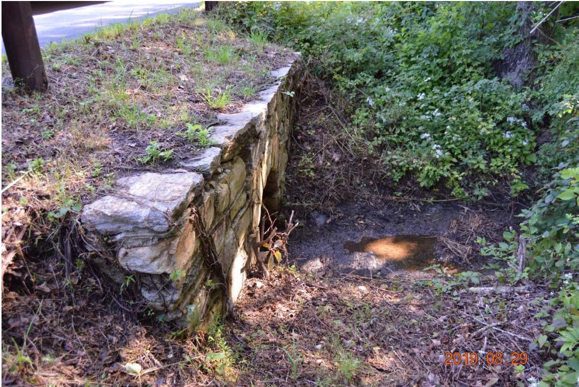
Photo 19e – The downstream end of the left side outlet pipe. This endwall is also in good condition.
