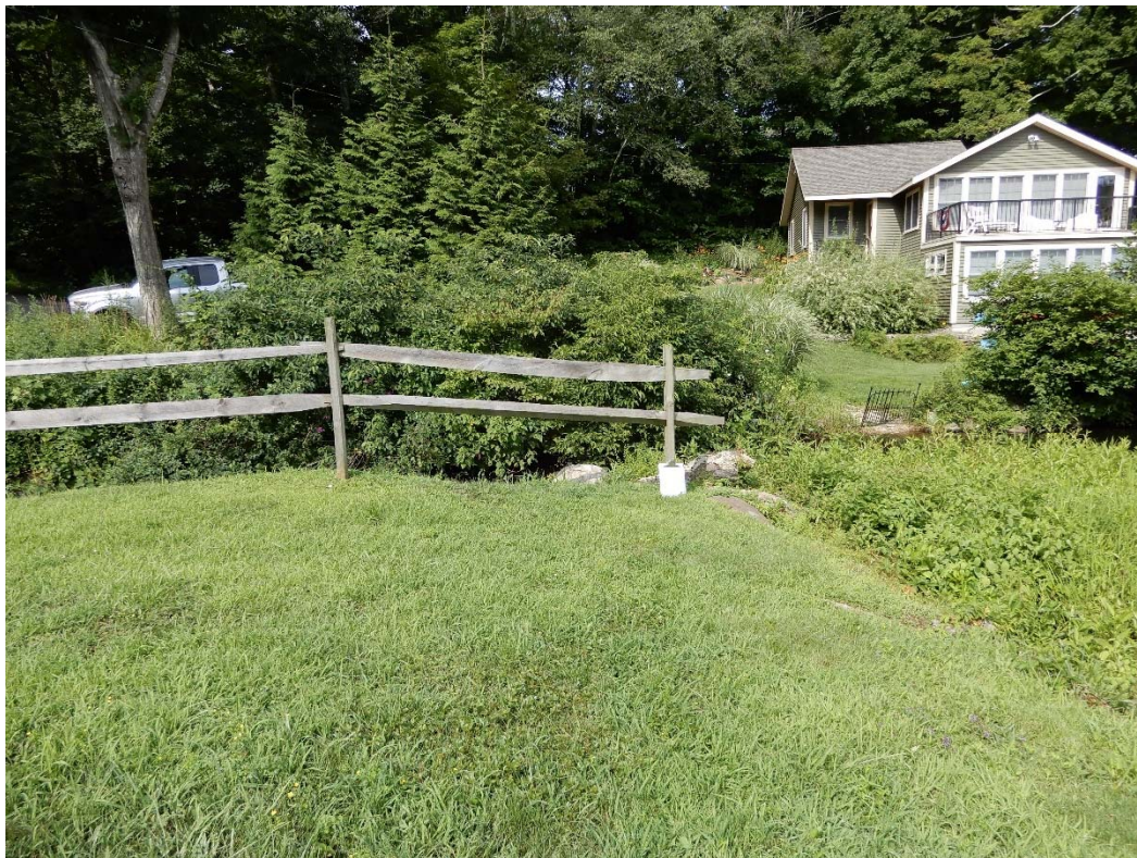
Photo 3a – The right upstream embankment face, prior to removal of vegetation completed between the two inspection dates.
