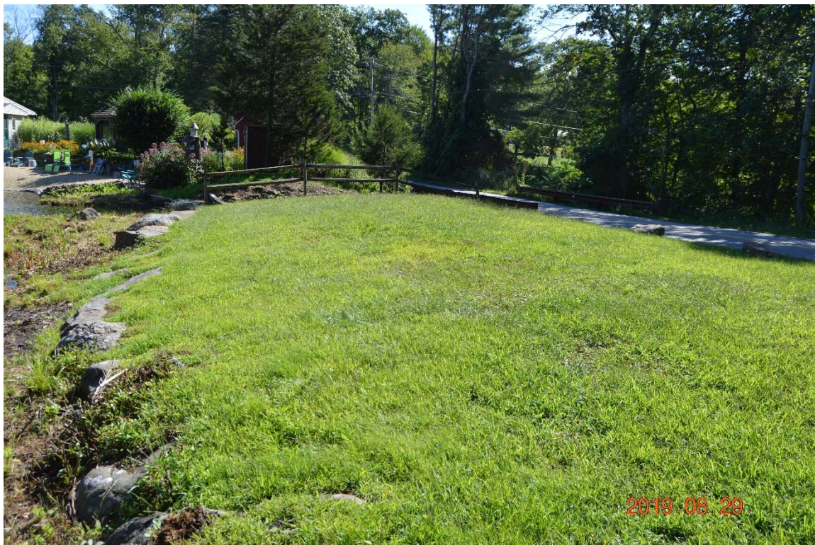
Photo 1b – An overview of Lake Hayward Dam from the right upstream side.
