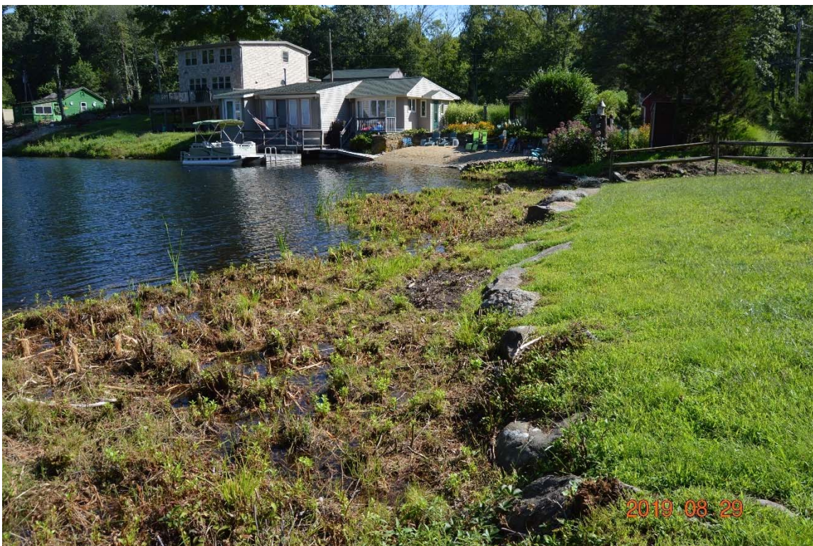
Photo 3c – Looking eastward over the upstream embankment from the right side, with vegetation removed, during the second inspection.
