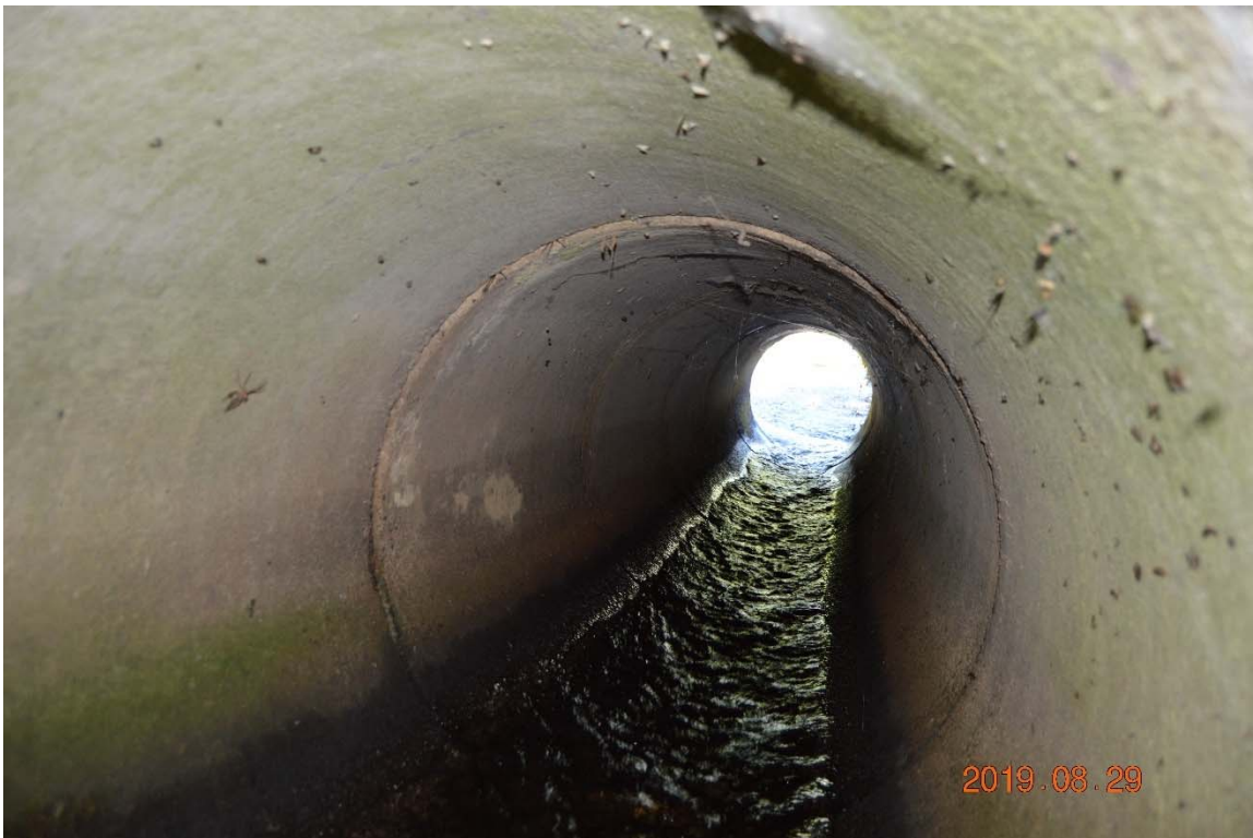
Photo 19d – The interior of the left of the twin right side outlet pipes, in good condition and representative of both pipes.
