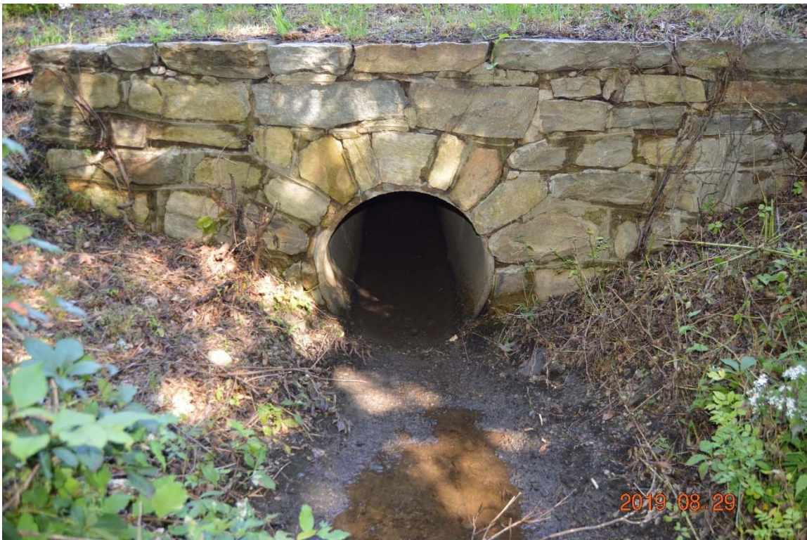
Photo 19f – A close up view of the downstream face of the left side discharge pipe.
