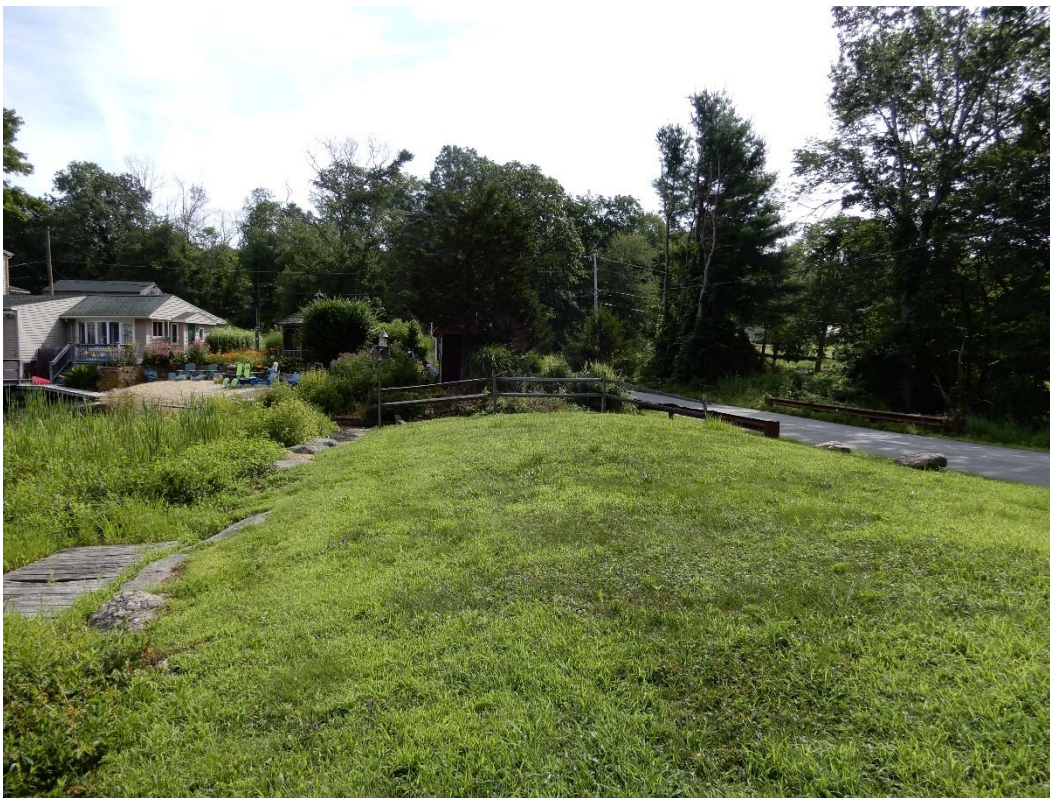
Photo 5a – The embankment crest as seen from the right side spillway area.
