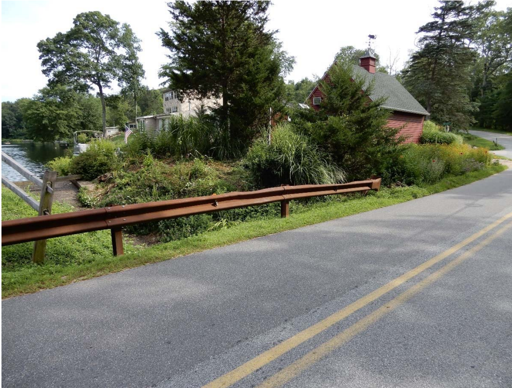
Photo 8b – The left side downstream embankment face (to the left of the left side spillway), prior to the removal of brush and vegetation.
