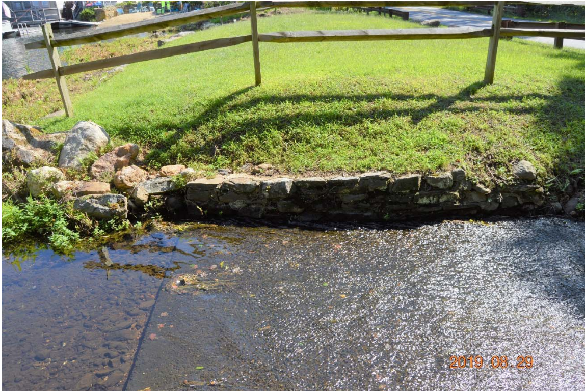
Photo 11b – The upper portion of the left side channel wall, again for the right side discharge channel.
