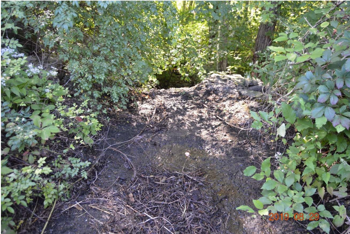
Photo 15f – The left side discharge channel stretching away beyond the apron at the base of the outlet pipe. At the upper center of the photo is a retaining wall from the old mill site, with a drop to the base channel of about 8 – 9 feet.
