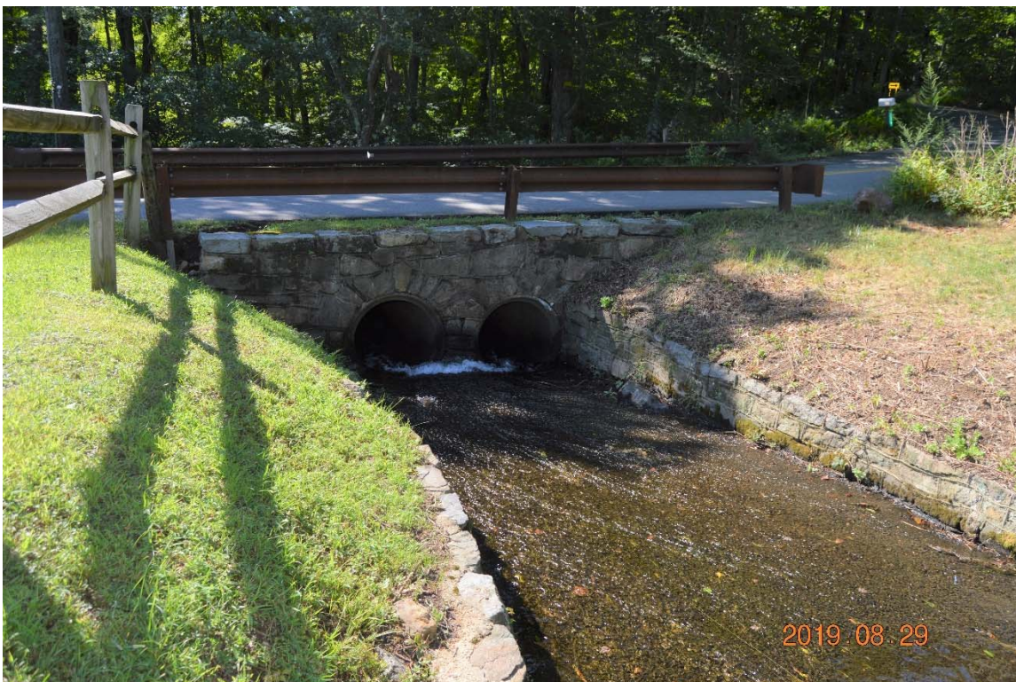
Photo 15c – An overview of the right side discharge channel as seen from the upstream side, following the removal of brush from the right side embankment. Note the two barrel culvert at the downstream end of the channel.
