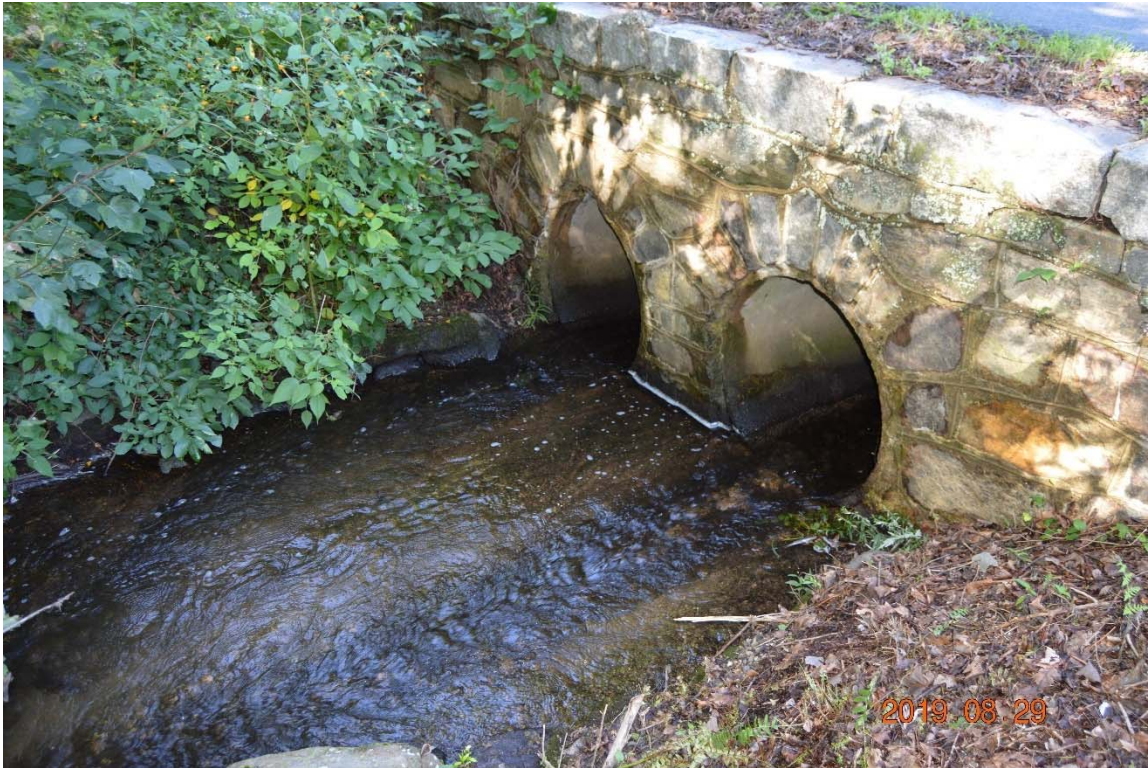
Photo 19c – The downstream end of the right side outlet pipes. The endwall is in good condition.
