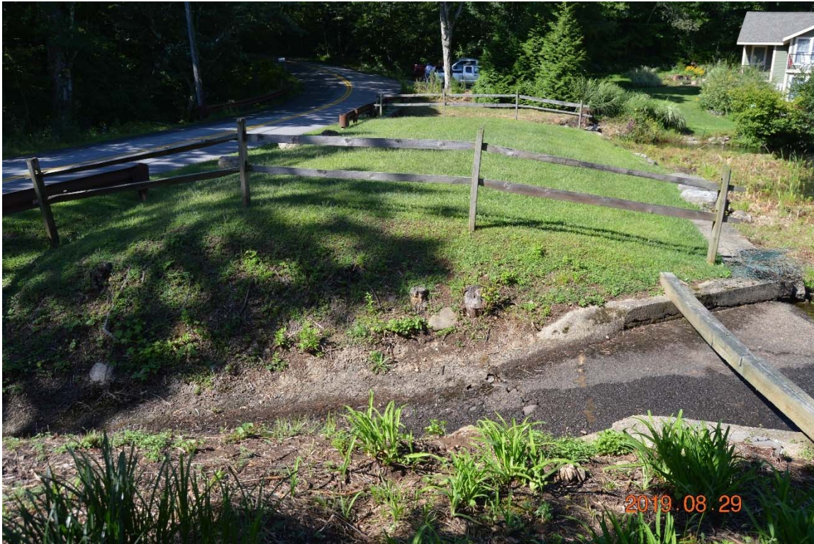
Photo 6b – Looking through the fence for an overview of the embankment crest as seen from the left abutment.
