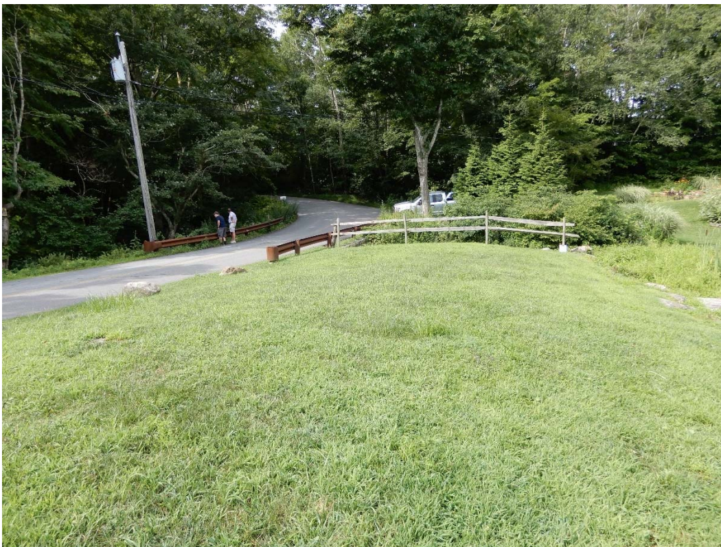
Photo 6a – The crest of the embankment as seen from the left side.
