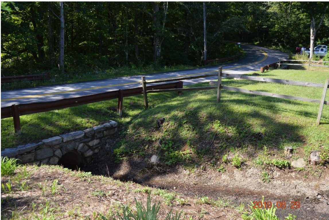
Photo 8c – Another view of the downstream embankment taken from the left side, with the transition to the left side discharge channel in the foreground and with tall vegetation removed.
