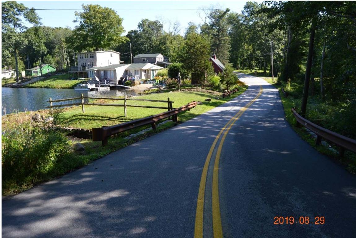
Photo 2 – An overview of the dam as seen from the road, to the right and downstream of the structure.
