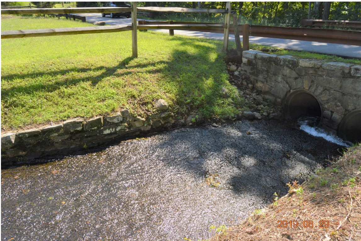
Photo 11c – The lower section of the left side channel wall for the right side discharge channel.
