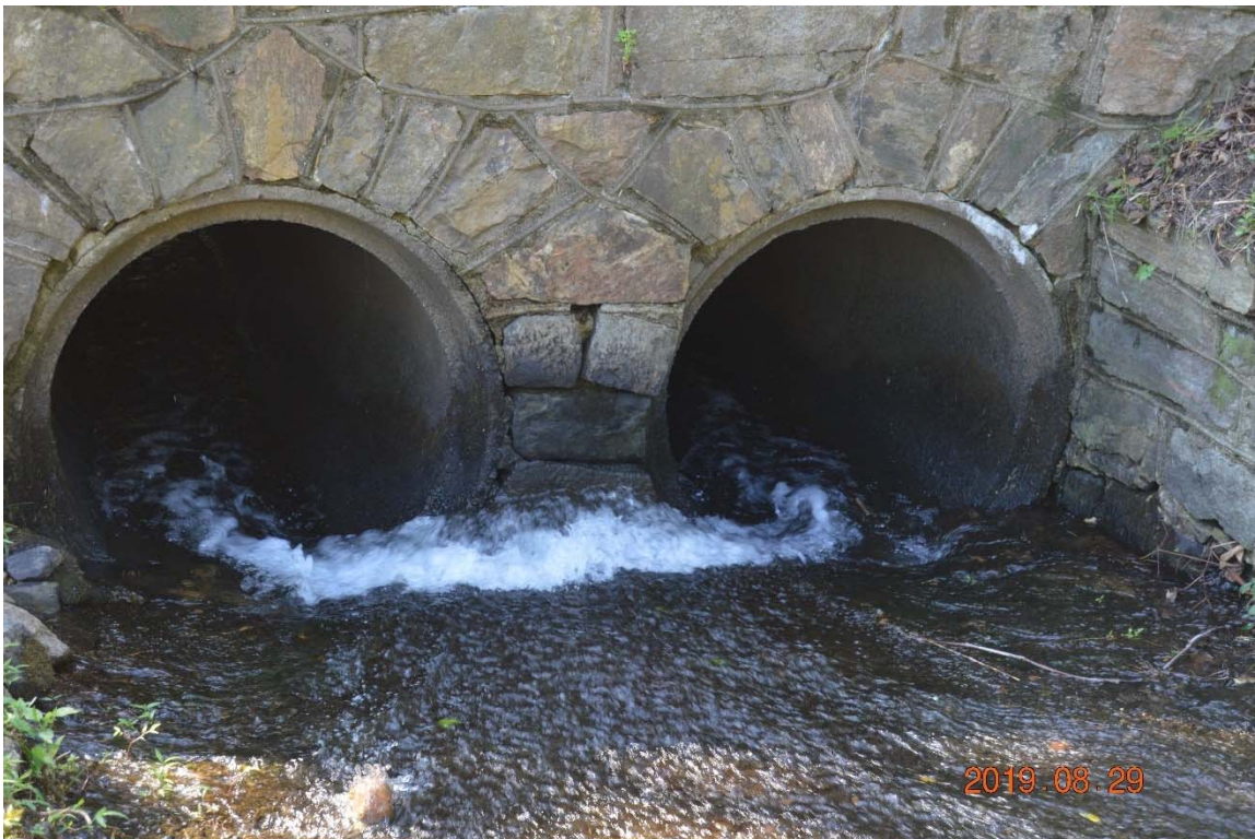
Photo 19h – A close up view of the upstream face of the right side discharge pipes.
